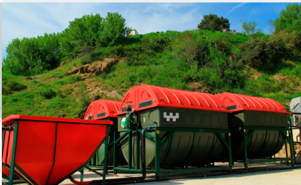
PlanetDISK® plant for 2000 pe at service of small community, Igneada Village, Blacksea region of Türkiye.
